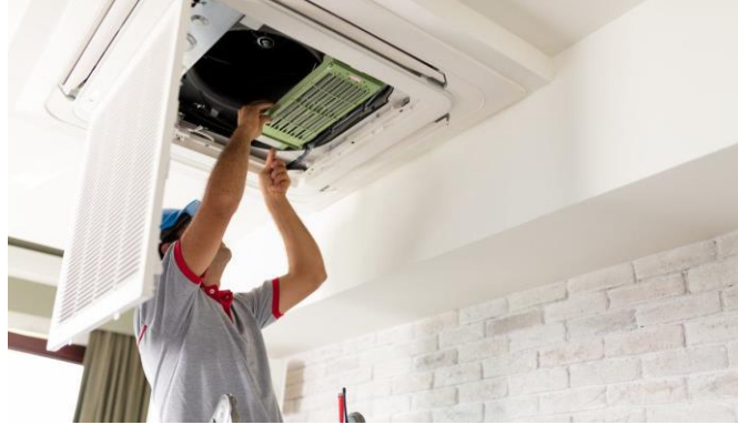
Figure 3 Technician maintaining AC [4]
