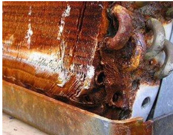
Figure 16 Corrosion on AC Coil [18]
